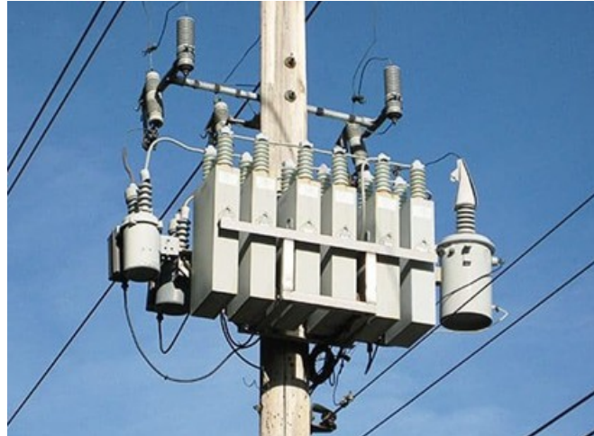
Power Factor Correction Capacitor Bank
