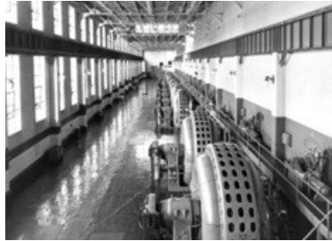
Schoellkopf 3-A Generators (The turbines were on the other side of the center wall.))
