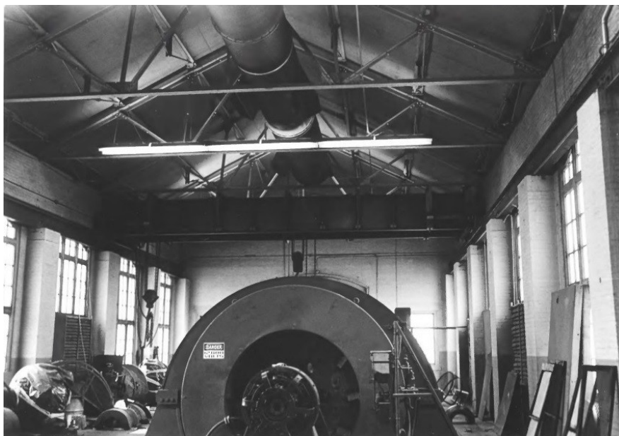
Transformer House Interior & Frequency Changer
