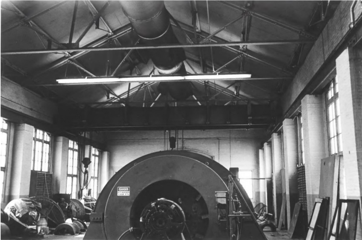
Transformer House with 60 Hz to 25 Hz Frequency Changer, a.k.a., Rotary Converter post-1940
